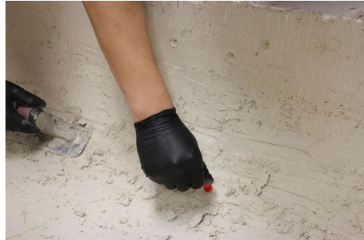
Figure 7. QC/QA member measuring the depth of a concrete layer on casting day.
