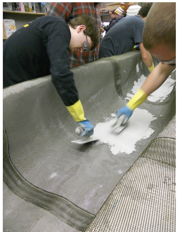
Right, the second layer of concrete is being placed. Concrete was placed over the first layer of reinforcement and then was troweled to the correct
