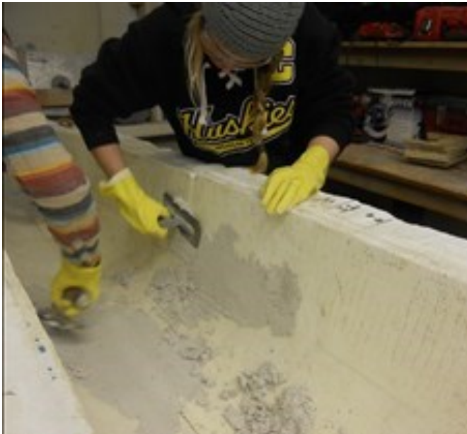
To the left, the troweling team places the first layer of concrete
