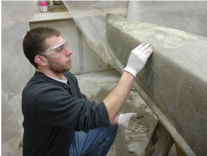
The interior and exterior of the hull were treated with finishing and slurry mixes to fill in any minor defects that were found.
