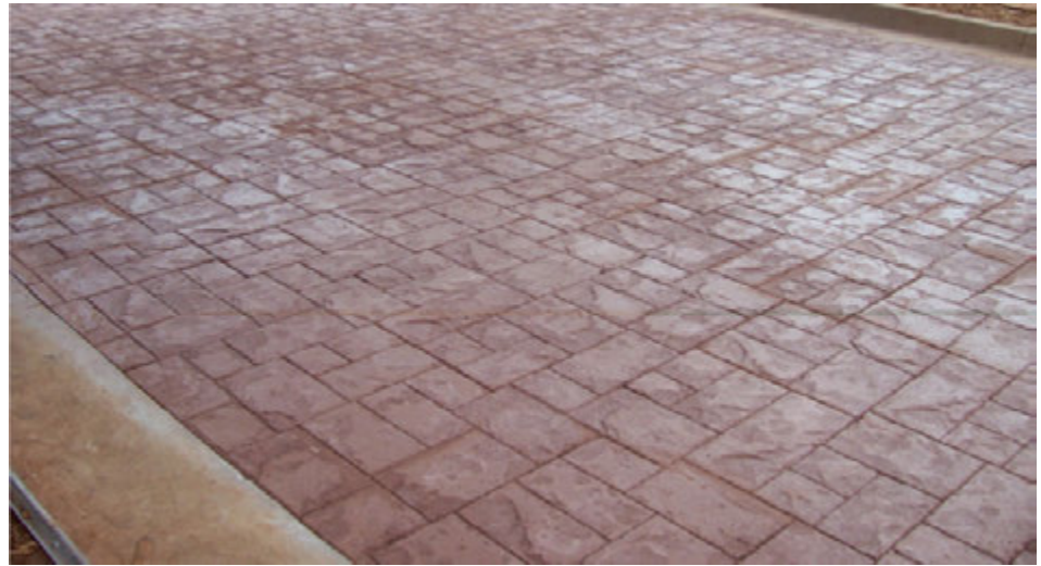
1835 Pigment in Stamped Concrete (Photo Courtesy of Decocrete)
